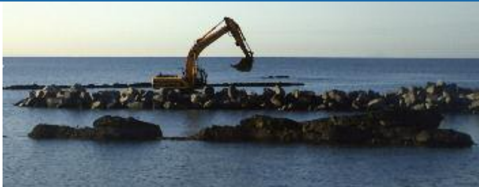
A view of the outer breakwater under construction in a gap between geological features of interest within the SSSI. Photo by E. Alice Johnson
