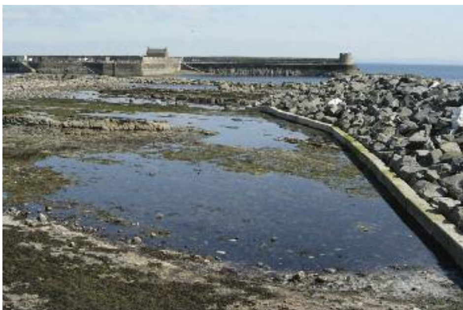
The finished outer breakwater. Impact upon the key geofeatures and contextual exposure has been kept to a minimum by breakwater location and method of construction.
